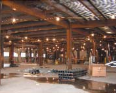
Future home of the Cardiac Catheterization and EP labs on the third floor of the new Van Elslander Pavilion.
