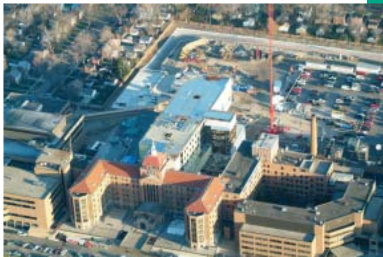
Aerial view of new Van Elslander Pavilion under construction (large white portion behind steeple in middle). (Photo by Gerald Donnelly)
